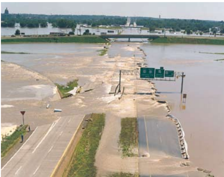
The Great Flood of 1993 caused flooding along 500 miles of the Mississippi and Missouri river systems. The photo shows the flood's effects on U.S. Highway 54, just north of Jefferson City, Missouri.
